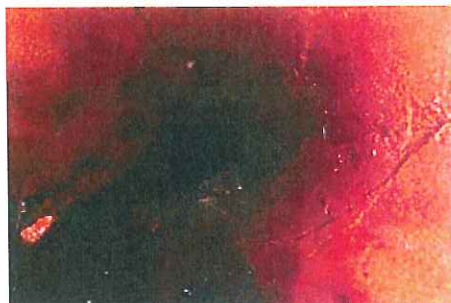
Figure 2 - Collapse Pipe (XP) Defect
