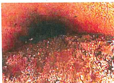
Figure 6 - Deposits Settled Compact (DSC) Defect
