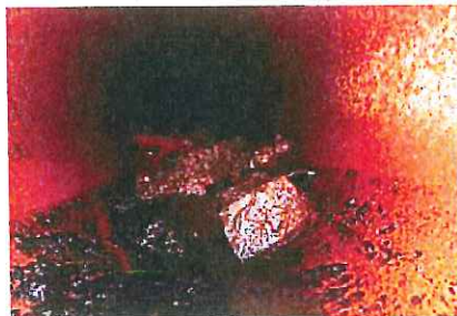
Figure 5 - Deposits ingress Settled (DNZ) Defect
