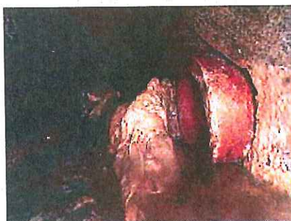
Figure 9 - Tap Break-in Intruding (TBI) Defect
