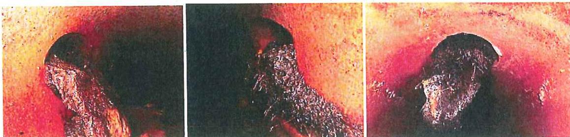
Figure 17 - Lateral Root Intrusion
