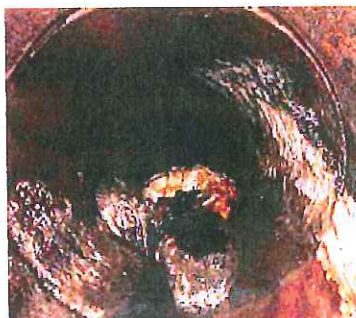
Figure 7 - Deposits Settled Other (DSZ) Defect
