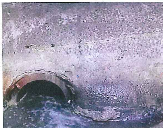
Figure 11 - Early Concrete Deterioration
