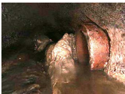
Figure 8 - Tap Break-in Intruding (TBI) Defect
