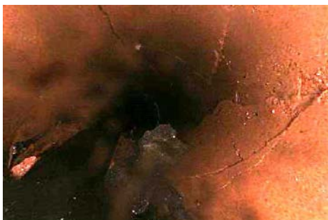
Figure 1 - Collapse Pipe (XP) Defect
