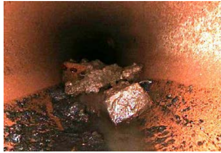
Figure 4 - Deposits ingress Settled (DNZ) Defect
