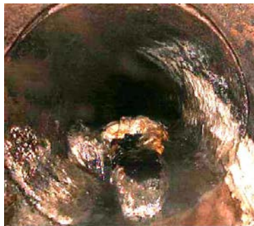
Figure 6 - Deposits Settled Other (DSZ) Defect
