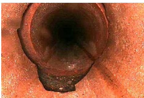
Figure 3 - Hole Soil Visible (HSV) Defect
