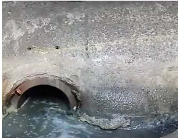
Figure 14 - Early Concrete Deterioration
