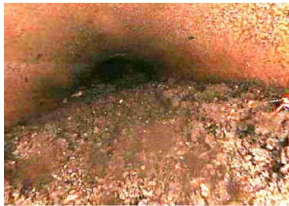
Figure 5 - Deposits Settled Compact (DSC) Defect
