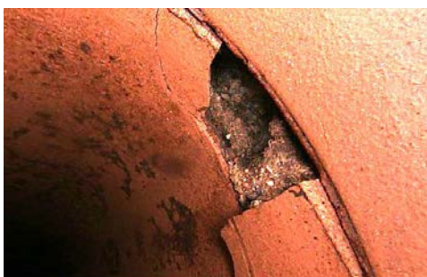
Figure 2 - Broken Soil Visible (BSV) Defect
