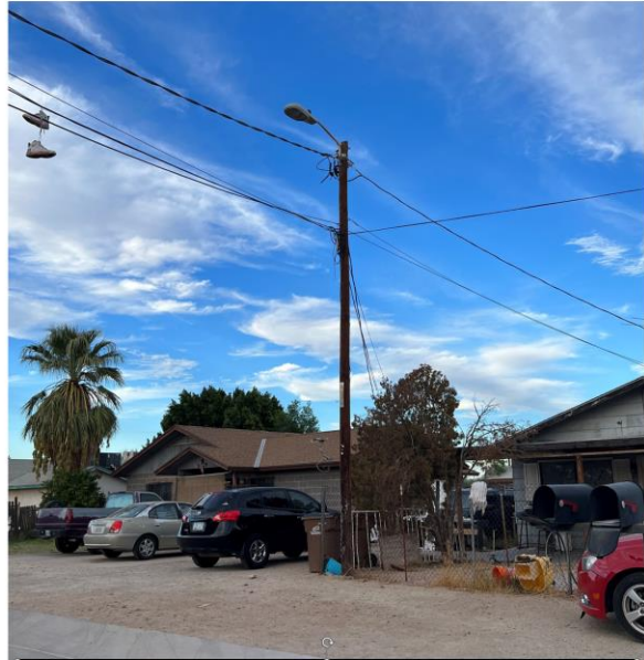
Calle Maravilla Cuarenta Area Neighborhood Town streetlight on SRP Pole
