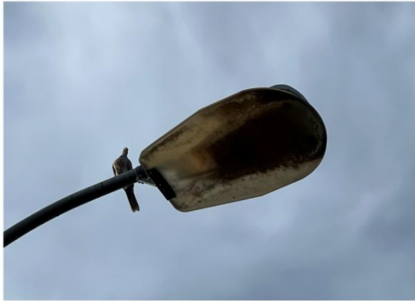
SRP Style Vandal Shield on Town Streetlight Protects the fixture, but if not cleaned Periodically will interfere with light delivery Cuarenta Area Neighborhood
